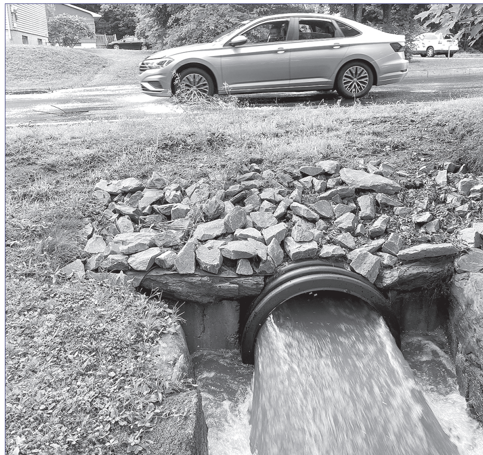
Excessive rainfall in Bridgewater, N.S., in July 2023 resulted in much flooding and damage to infrastructure.
